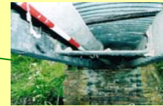
Pipe passing under the Chapel foot-bridge, Brownhill Creek
